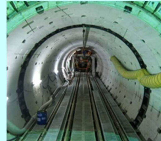
Horikawa -river left bank Rainwater Reservoir for pollution control
