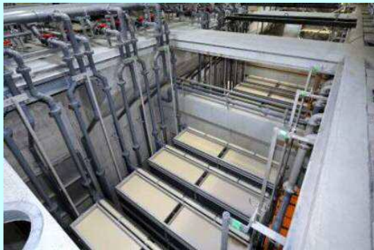
Flat membrane unit aerobic tank
