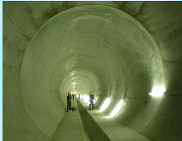
Started operation in 2010 (13,000m 3 )
